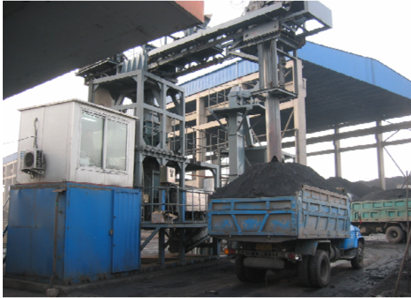
Coal Truck Auger Sampling System
